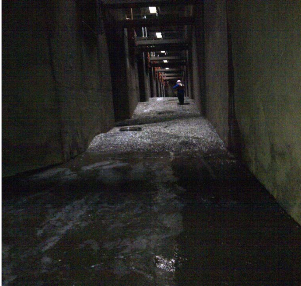
AWS channel accessed for EFL backup water supply study. Approximately 6' depth clam shell buildup at one location. No major flow restriction concern, thus no plans for removal.
